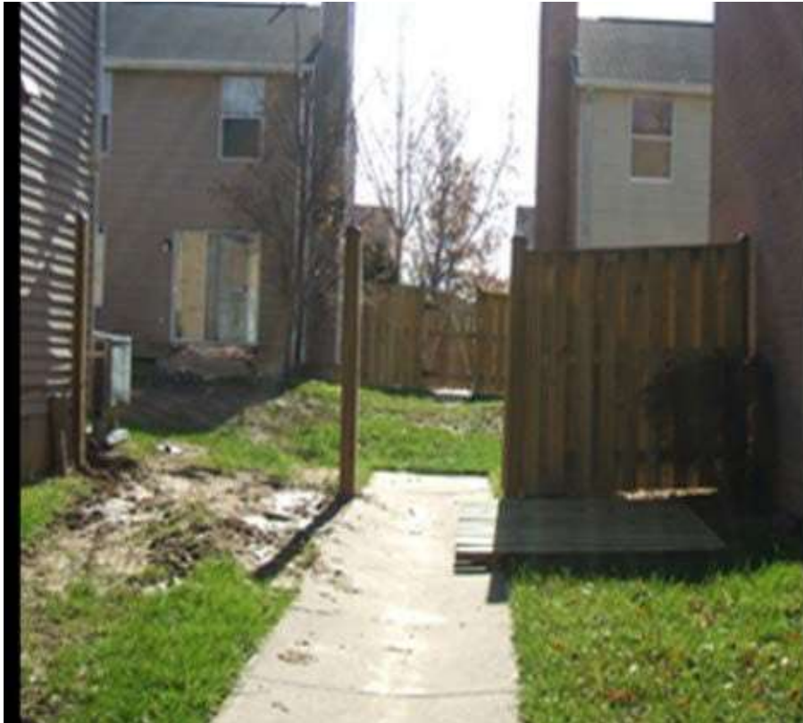
Unable to see through the property: Blind spots behind the fence offering concealment to the criminal element.
